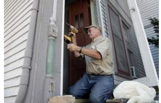
Duwayne Krause of Consolidated Construction Co. works on the home of Debbie Nelsen of Appleton. Post-Crescent photo by Kirk Wagner
